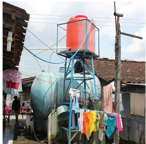
A public hydrant distributes water to families in a dense low-income community in Semanggi.
